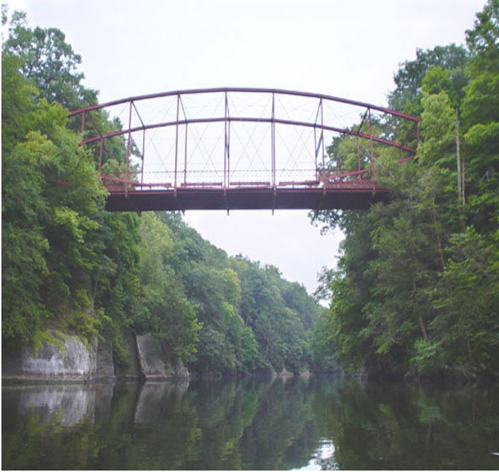
Figure 4 The Berlin Iron Bridge Company's lenticular truss bridge over the gorge at "Lover's Leap"
